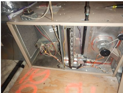
Blower compartment cover removed
