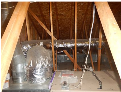
Ductwork in attic
