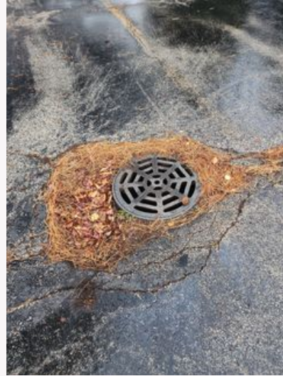
Settling at drain basin in parking area
