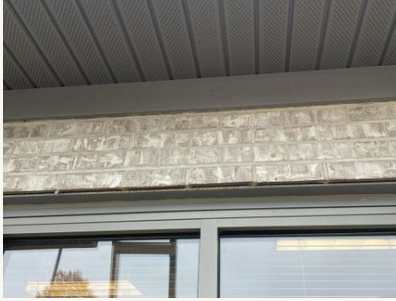
Rust at lintel (typical many areas)
