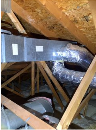
ductwork in attic space
