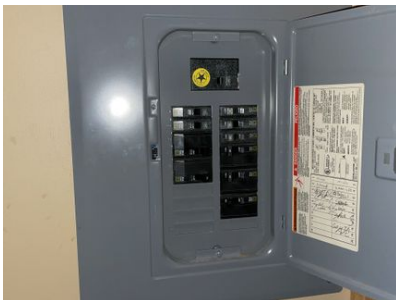
Suite A Sub Panel
