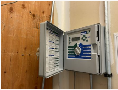
timer for sprinkler system
