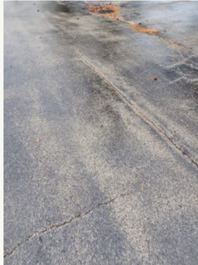
Typical cracking of parking area
