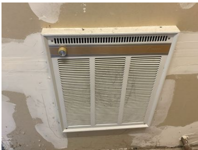
Storage closet wall heater
