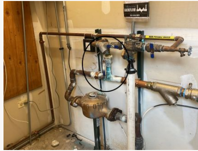
note stains and corrosion at backflow preventer
