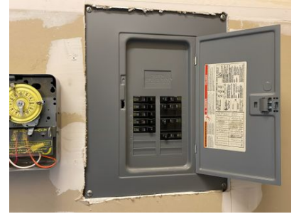
Common Area Electric Panel
