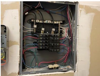
Common Area Electric Panel Interior
